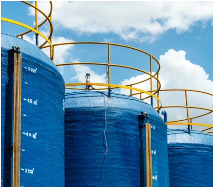
Capture water level in storage tanks.
